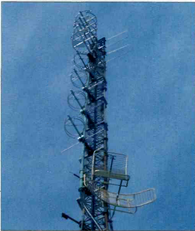
WNNK, Harrisburg, PA, has an interleaved antenna system (upper antenna) mounted directly above a backup antenna.
