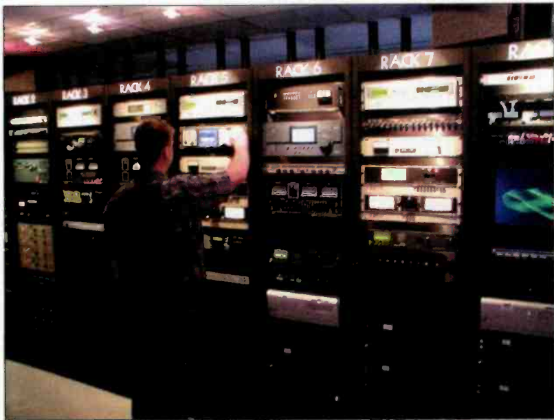
Greg Trobridge checks the processing in the rack room, which is a showcase in itself with its clean layout and aesthetic lighting.
