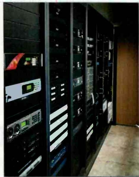
The equipment racks face a glass wall so visitors can see the backbone of the station.
