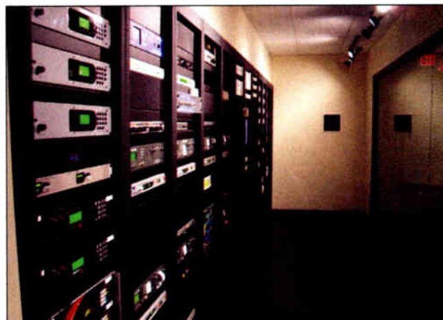
Station visitors can view the outer terminal equipment rack room through a window. The entire rack room is 1,100 square feet and is compartmentalized into three distinct areas.
