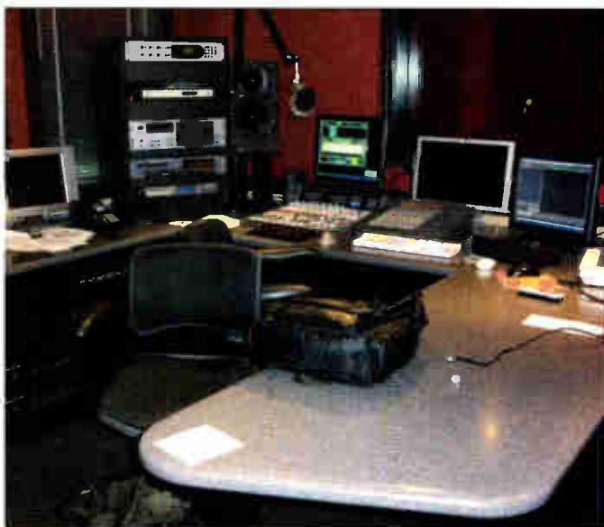
Production 2, centered around a Wheatstone G-6 with the Audio Vault, Pro Tools and DAW screens, faces into the voice over booth.
