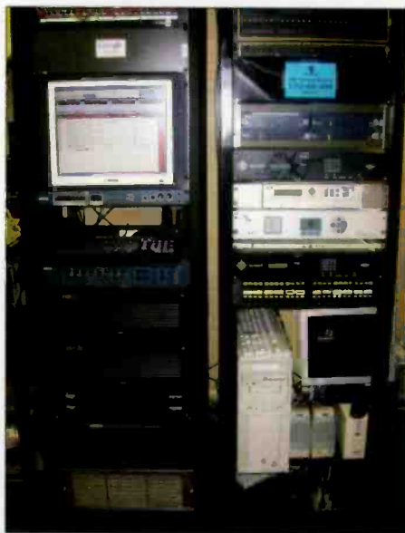
Equipment racks in central engineering, containing Maestro Automation on the left and satellite equipment on the right.
