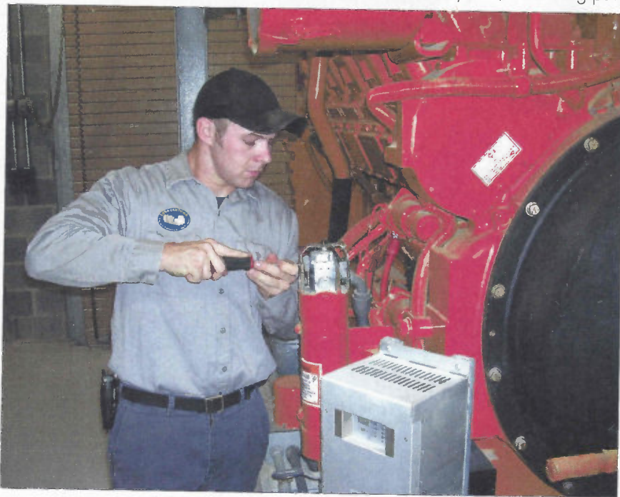
Generators are available in sizes ranging beyond 10MW.
