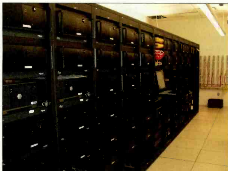
The 14 racks house the audio storage and playback system.
