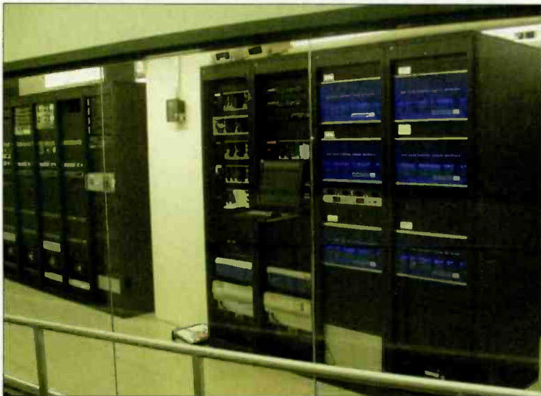
The master control room is visible through a glass wall.
