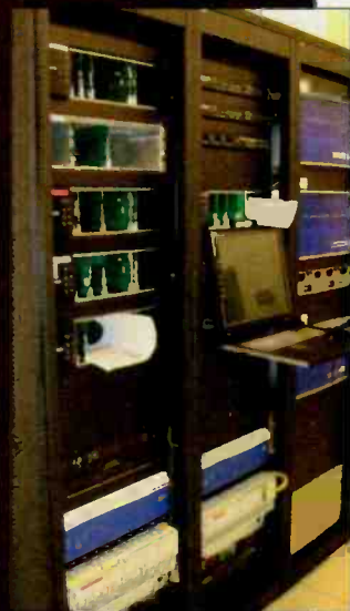
The transmission rack is the hub of feeds from the station to their transmitter sites.
