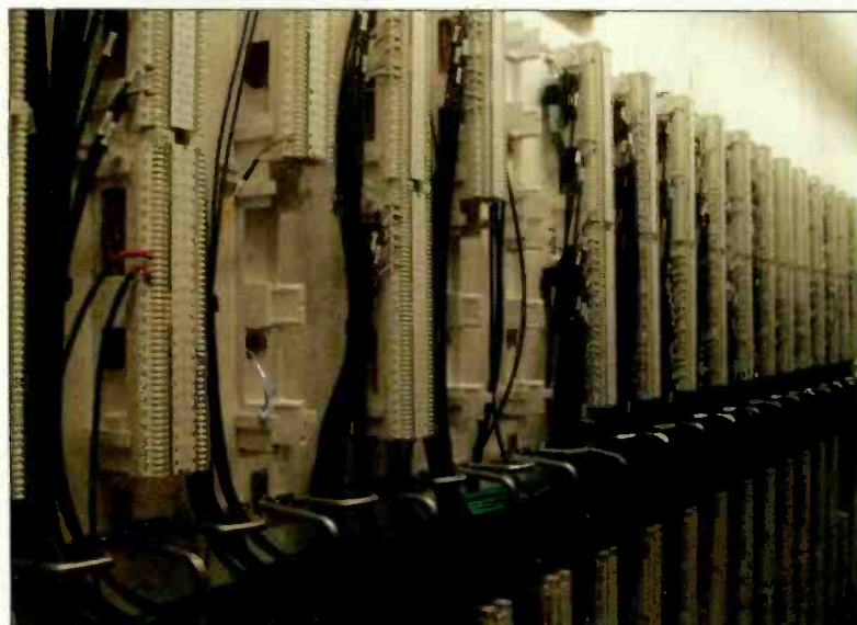
Krone blocks form the heart of the facility infrastructure.
