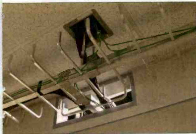
A wire tray exits the TOC feeding individual studios through square cable chase conduits.
