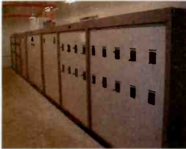
CUSTOM PHASOR INSTALLATION
