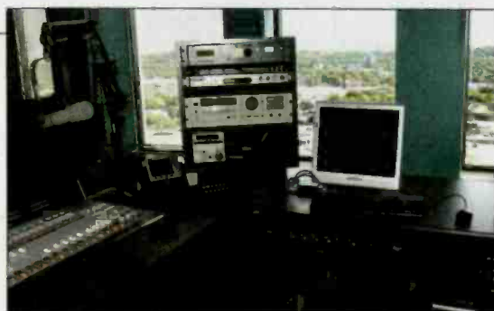
Large windows allow plenty of light into the Wdvi control room.
