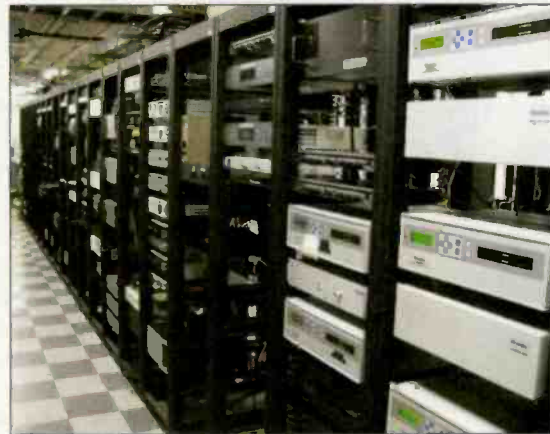
All lined up in the rack room.
