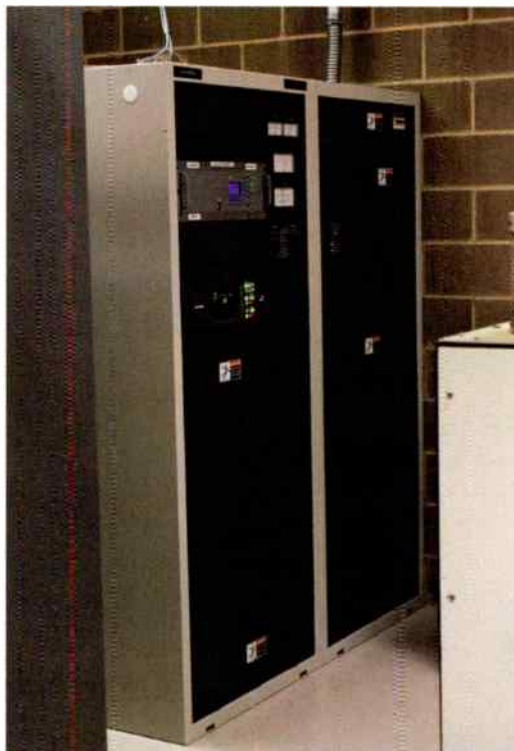
KHCC: HPX40 that will be partitioned off from the room to allow ventilation of the cavity from behind. This will cut cooling requirements drastically.
