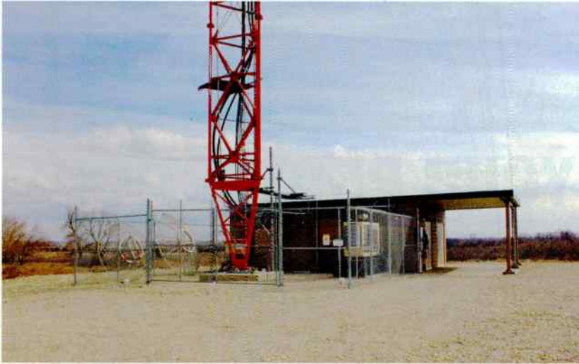
KHCC's building includes spare 950MHz antennas and an 80kW diesel generator.
