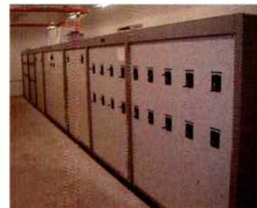
CUSTOM PHASOR INSTALLATION
