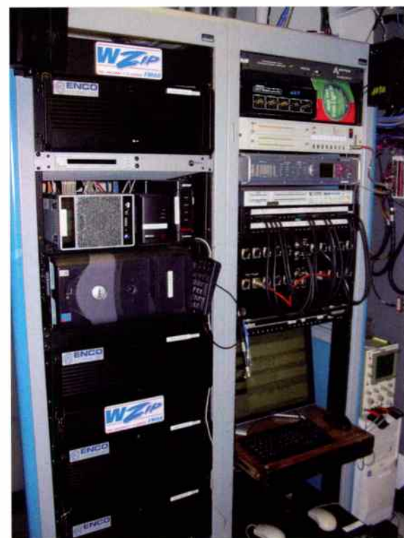
The computer and wiring interconnect room houses the Enco workstations, Buffalo and Netgear NAS servers, Telos Profiler and Invonics modulation monitor.
