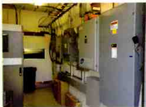
TX site electrical system
