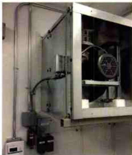
Economizer system at TX site
