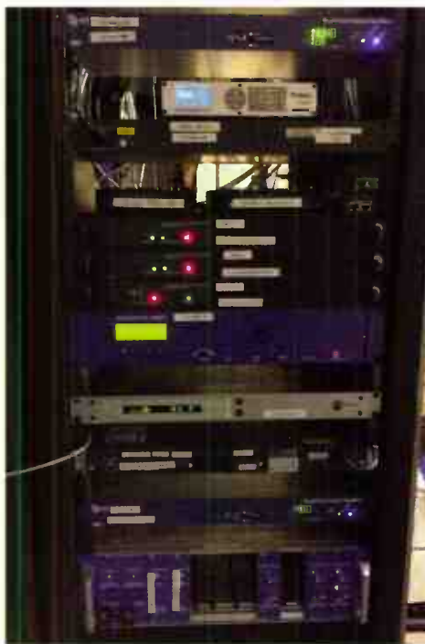
KBXE Engineering rack and audio codecs
