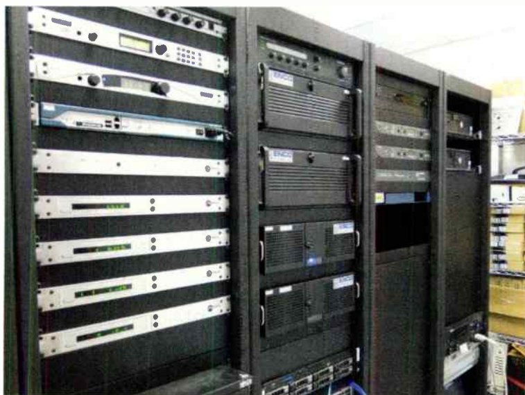
The technology center houses support equipment for the studios.
