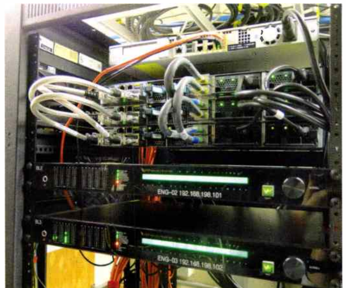
WheatNet switch and Blades in the rack room provide an AoIP STL
