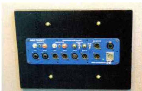
A Henry Engineering “Multiport” panel allows quick access to audio and network I/O.
