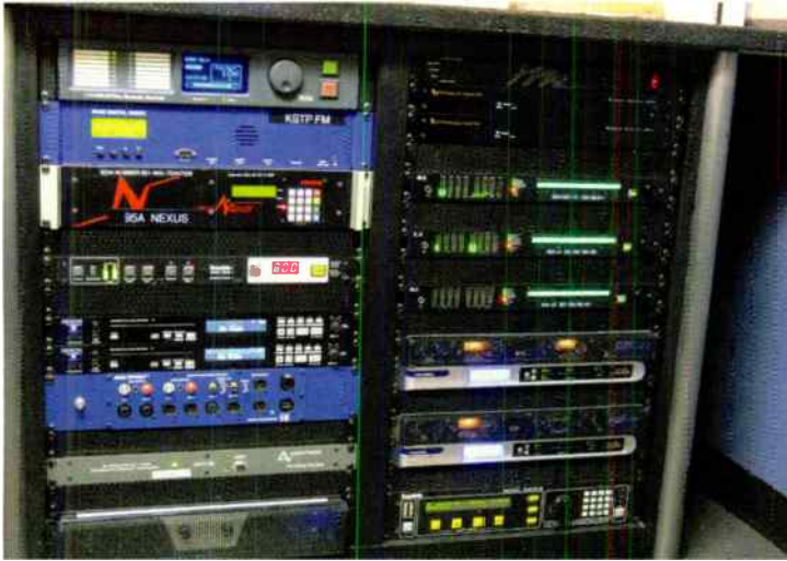
Racks for equipment that does not require immediate operator access are tucked out of the way, integrated with the furniture.
