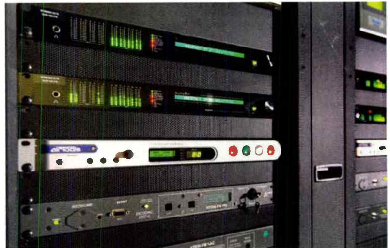
Wheatstone Blades in the TOC handle audio and logic I/O from each station's airchain and other equipment.
