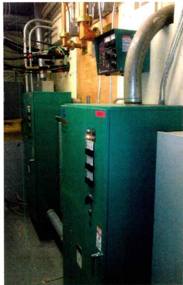
Figure 5: Redundant Automatic Transfer Switches
