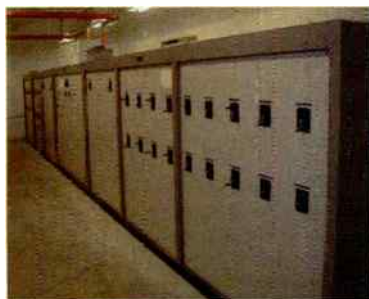
CUSTOM PHASOR INSTALLATION
