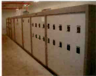
CUSTOM PHASOR INSTALLATION
