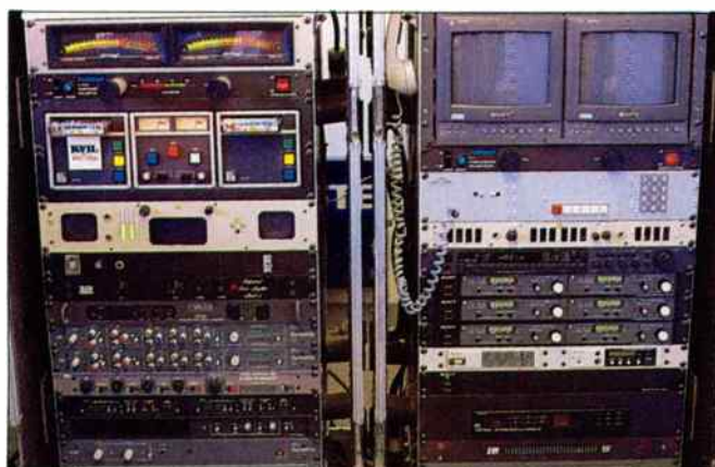
Two rolling vertical racks contain most of the audio and RF equipment that goes into the control booth.
