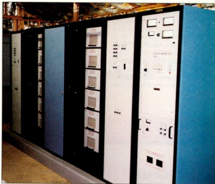
Solid-state transmitters are less demanding in their cooling airflow needs.
