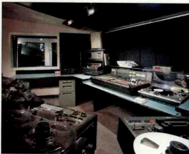
Control rooms at MJI allow simple reconfiguration for integration of future technologies.
