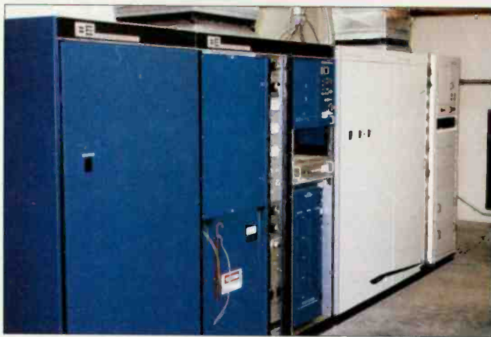
Proper ventilation is important to any transmitter's longevity.
