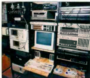
Some of the equipment in the EIA's DAB test van.
