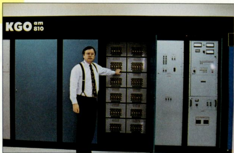
KGO-AM's director of engineering Bruce Schirmer with one of the station's two Nautel ND50s.
