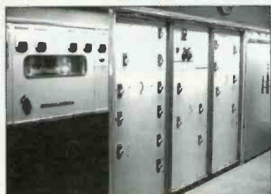
AM WIDEBAND DIRECTIONAL ANTENNA PHASING SYSTEM
