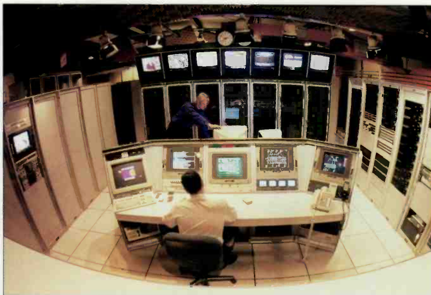
Uplink control rooms like this one at Chicago International Teleport handle many reports of reception difficulties, but they can't do much when the problem comes from a downlink's receive antenna.
