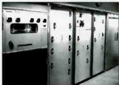
AM WIDEBAND DIRECTIONAL ANTENNA PHASING SYSTEM
