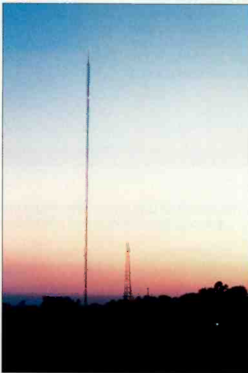
Tower light maintenance is the responsibility of the owner. (Photo by Chriss Scherer.)
