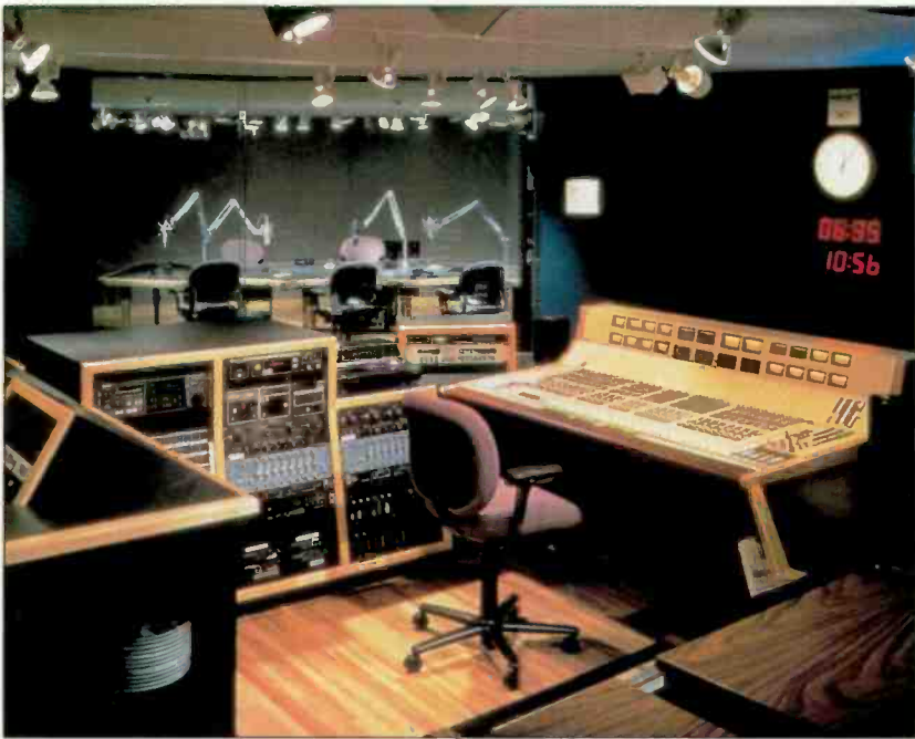
Specialized construction components are required to provide adequate sound isolation between rooms (doors and windows), and appropriate interior acoustics (absorptive wall and ceiling finishes). (NPR, Washington, D.C.)
