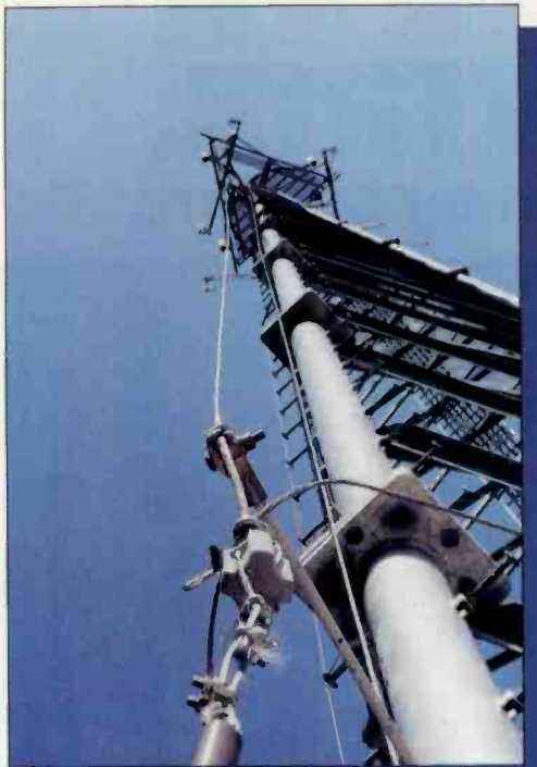
Detail of the PCS tower's detuning skirt. The cost of detuning was paid by the PCS companies.
