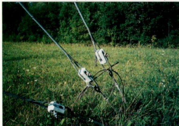
Some corrosion is forming on the turnbuckles. Maintenance is required.
