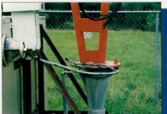
A typical maintenance problem. The bonds and bolted connections on this feeder must be physically tested and examined.
