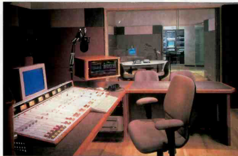
Control Room B, built around a Wheatstone A-6000, looks into Studio B. The Tech Center can be seen in the background (Position 1).
