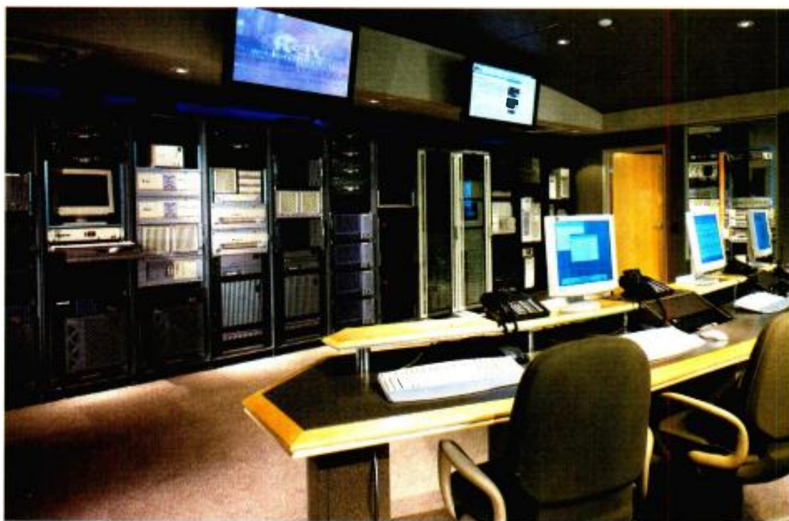
The Data Center & Web Hosting Facility provides both traditional web hosting services and serves as a new distribution channels for content and digital assets. Currently over 1400 web sites are supported from the operation.
