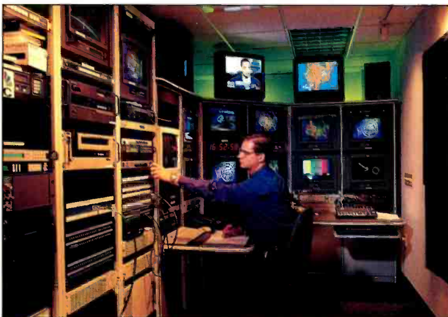
Master control for AccuWeather's WeatherTeam and WeatherTeam Live segments is equipped with a 16-input Grass Valley 1200 serial component digital production switcher.
