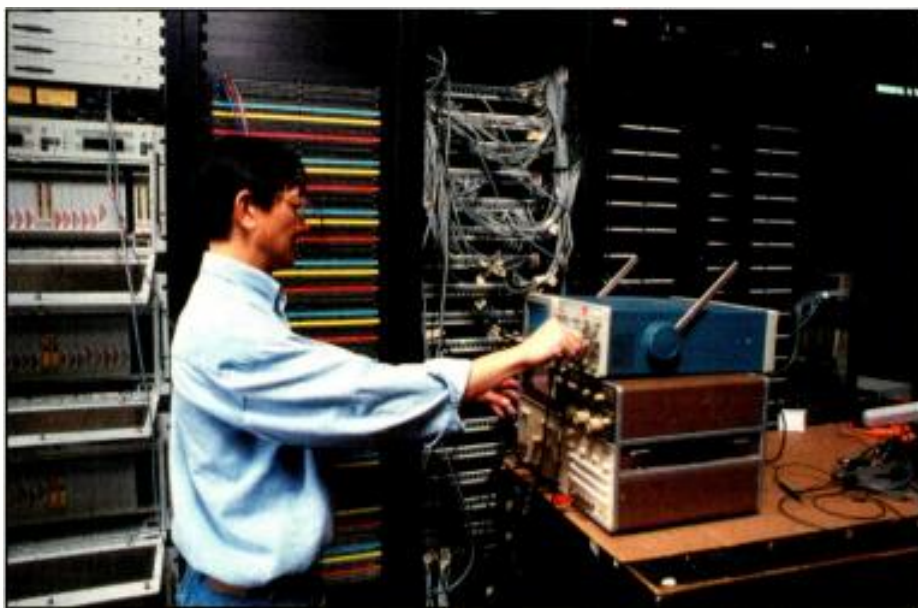
Telex's Willie Yau at work in the company's Lincoln, NE, facility, where the company worked closely with NBC to develop the intercom and communications systems component of NBC's "rack in a box" concept. Each "RIB" was a fully-wired subsystem loaded into one platform.
