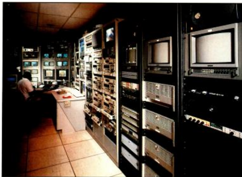
View of the new WVPT digital master control.
