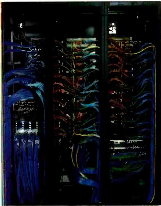
Rear view of routing rack.
