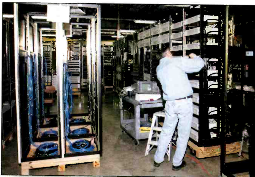
While final construction is still progressing, off-site equipment rack integration keeps the build process on schedule.
