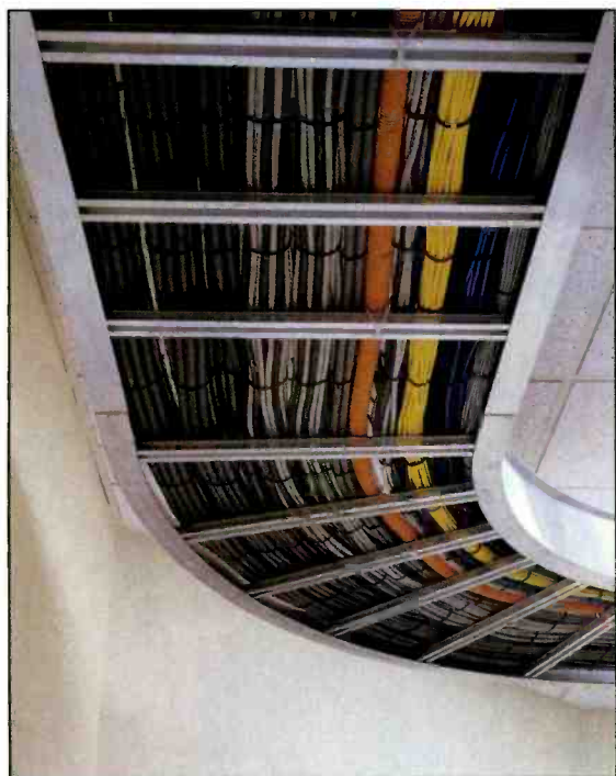
Careful planning results in convenient and attractive solutions to difficult facility challenges. This overhead cable tray is an accessible alternative to under-floor runs.
