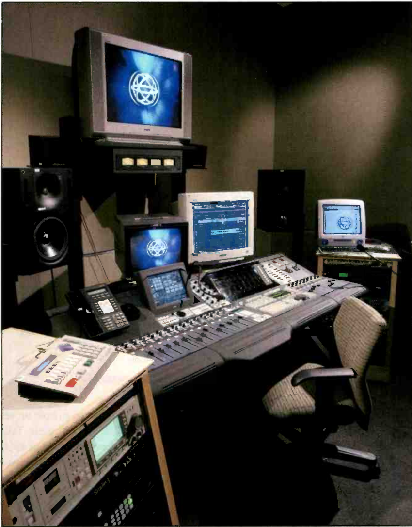
Turner Studios in Atlanta. Note the use of video monitors for audio applications. In such applications, be sure the monitors are properly shielded or you'll have more hum than with a bad cable. Also watch how close to the monitors microphones are mounted. The monitor's horizontal sweep circuits can create an audible high-frequency buzz if the mic is located anywhere close, especially if you are using low-quality displays. Photo courtesy Daniel O'Connell.
