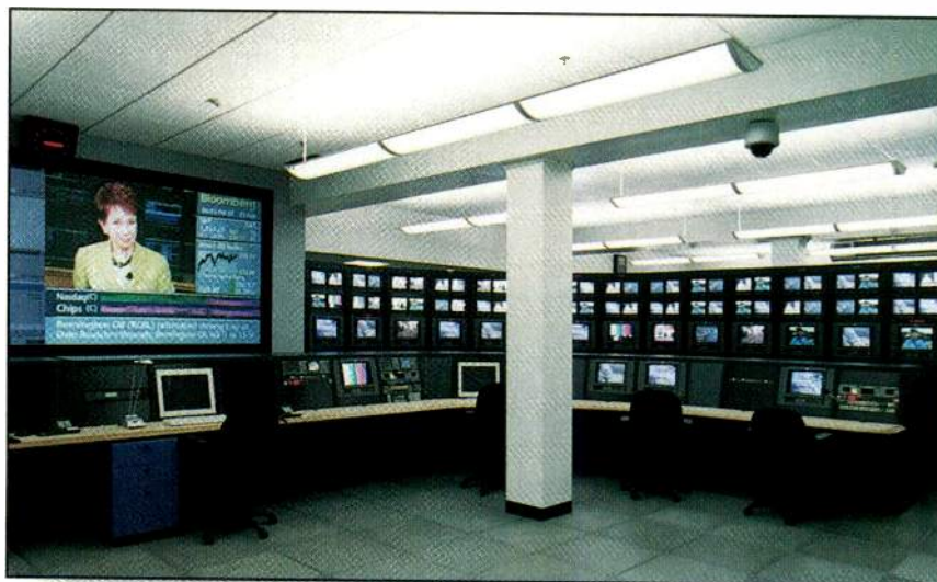
From the video monitoring and media wall in Activate's network and satellite operations center, operators monitor the progress of the signal within the facility, from ingest of incoming feeds through signal processing.
