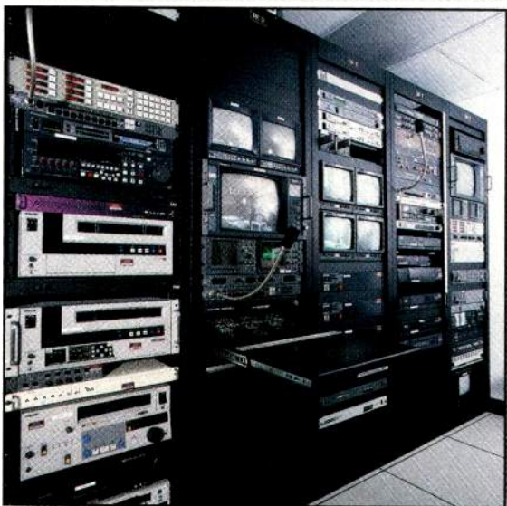
The main equipment room handles signal ingest, routing and patching in the new facility. Signals going to and coming from analog equipment are converted to digital to eliminate the need for special routing or patching.
