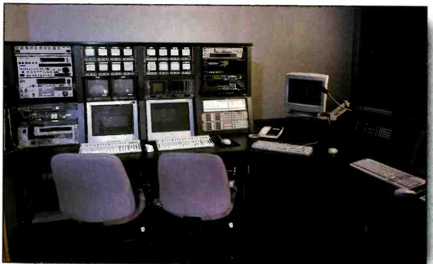
BlueLine's Station Master automation system controls the two channels that KJLA broadcasts.
