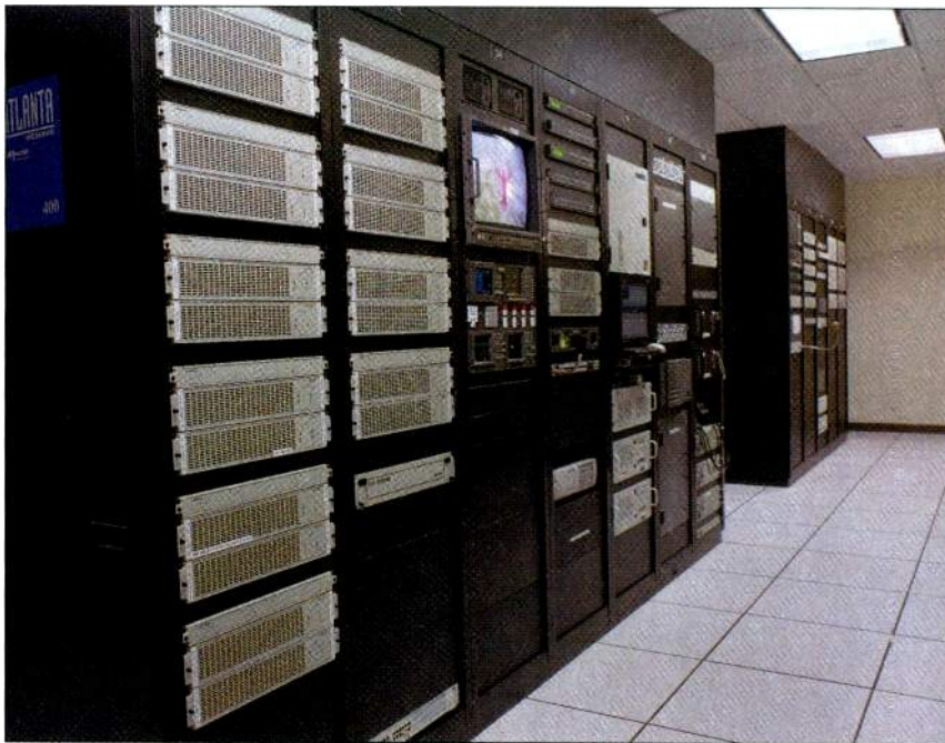
Conversion equipment and legacy systems at WGCL are located for easy replacement with digital machines in the future.
