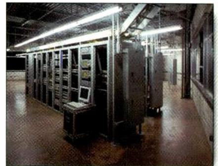
The design for the new media center includes extra rack space and router capability to accommodate growth in the company's IP- and fiber-based transmission services.
