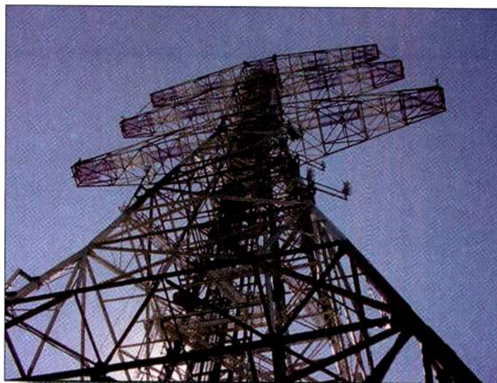
The Armstrong tower resembles more of an electrical power transmission tower than a broadcast one. The three horizontal arms were made for difficult broadcast antenna installations. The tower had been used primarily for two-way, land-mobile and cellular antennas.
