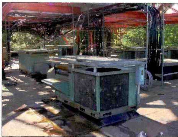
The evidence of low-power radio usage on the tower is evidenced by more than a hundred separate coax runs, as shown above.
