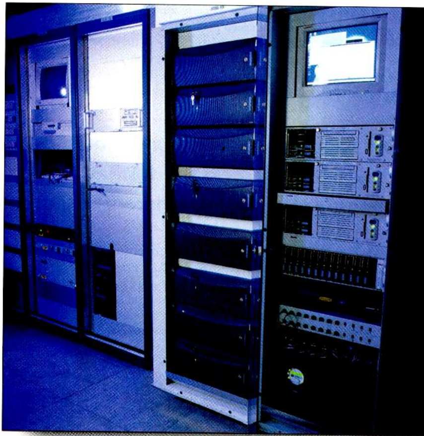
Four SGI Media Servers for broadcast (purple rackmounted systems) and RAID-3 storage by Ciprico provide dual redundant systems for newsroom and airplay operations at Danish Broadcasting.
