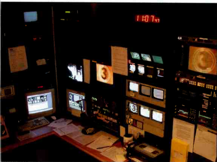
Transmission operations center (TOC). Microwave, STL, TSL, Satellite Fiber and ENG all pass through this center. Photo courtesy Telemundo.
