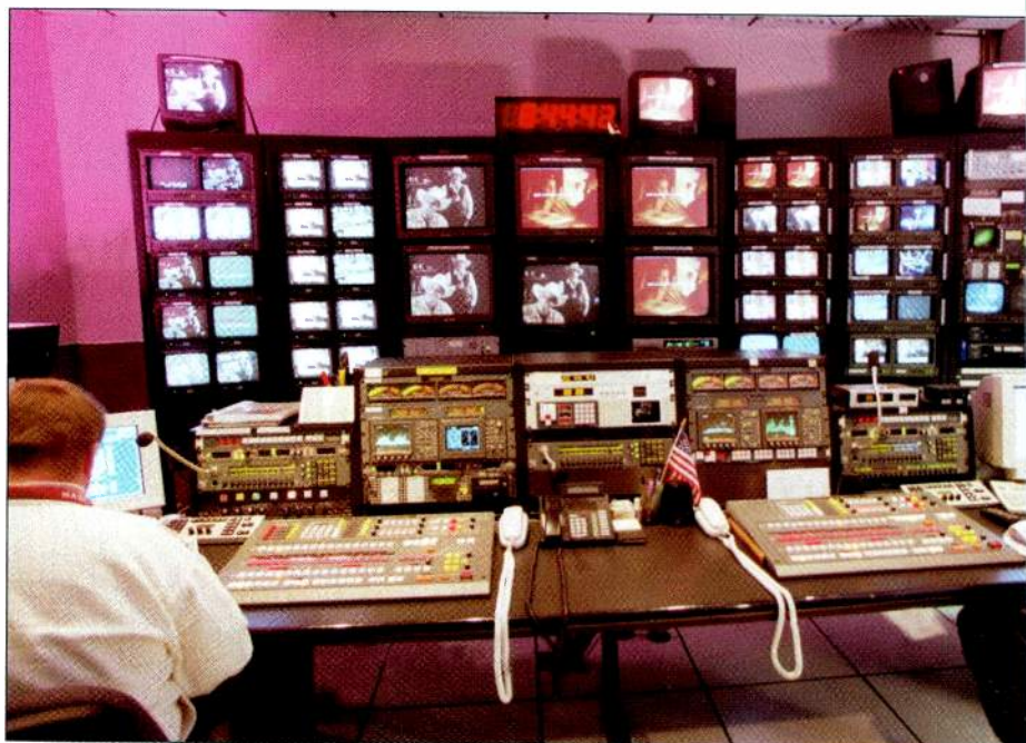
KVEA-TV/KWHY-TV master control with KWHY-TV monitors, switcher and other equipment on the left, and KVEA-TV, a mirror image on the right. Photo courtesy Teklogic.
