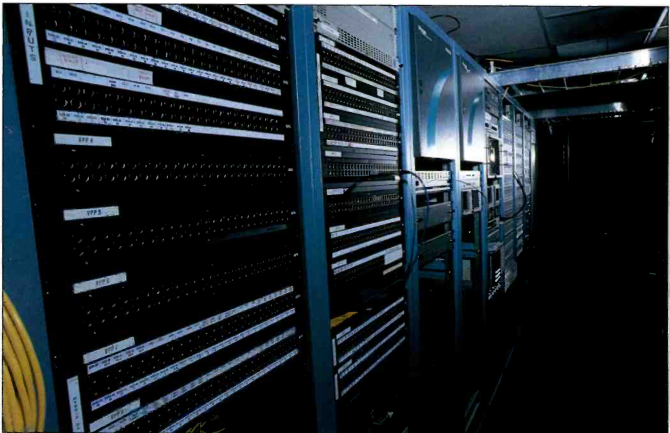
The central equipment room (CER) houses the routing equipment, master control switching equipment, audio and video distribution amplifiers, all of the production switcher frames, digital video effects generators, and the video servers.
