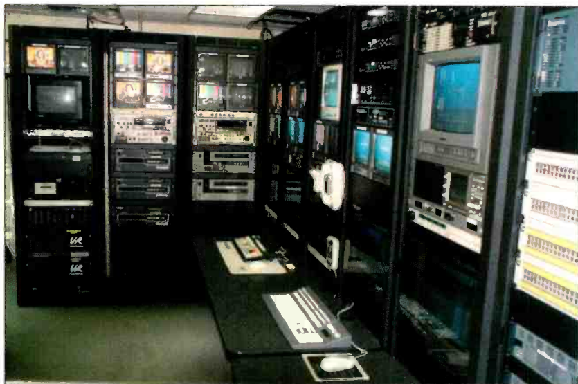
Prior to the re-build, KTYO was a manual operation using 3/4" tape machines. The challenge was to completely empty the existing MC and rebuild, while keeping the station outage time to a minimum.
