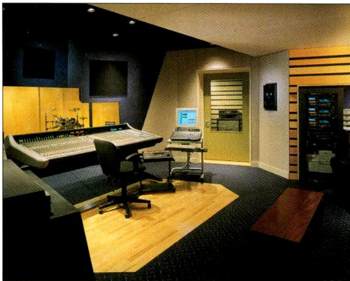
Control Room A at Egan Media Productions features a 64-input D&R Cinemix 5.1 console with moving fader automation, onboard dynamics, and 24-input STEMS film mixing module. Photo courtesy Egan Media.
