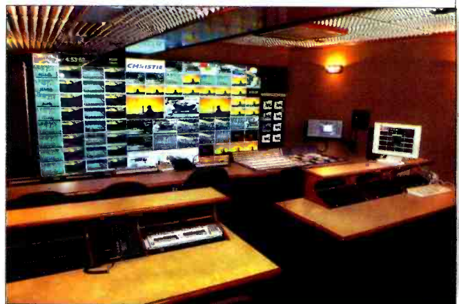
The virtual monitor wall in Core Digital/SWTV's new all-digital hybrid mobile television truck uses Avitech's Video Command Center (VCC) line of processors for monitoring up to 96 SDI sources on six Christie Digital 50-inch DLP cubes.
