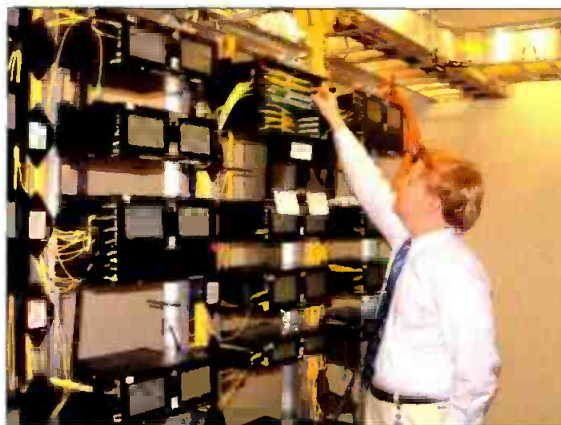
Rick Ackermans, director of engineering for Turner Entertainment Networks, examines the fiber-optic cross-connect facility in Turner's new six-story broadcast facility in Atlanta. The room contains over 600 strands of single-mode fiber and over 300 strands of multimode fiber.
