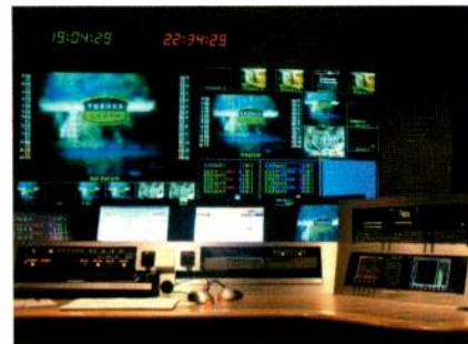
THE SOUTH CONTROL ROOM - ONE OF NINETEEN FEEDS AT THE NEW NETWORK OPERATIONS CENTER
