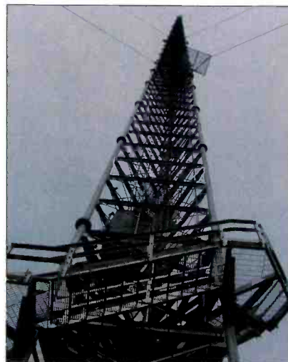
After struggling with aeronautical and station-spacing issues, KMOS selected a site 55 miles away from its Warrensburg, MO, studios for its new 2000-foot tower.
