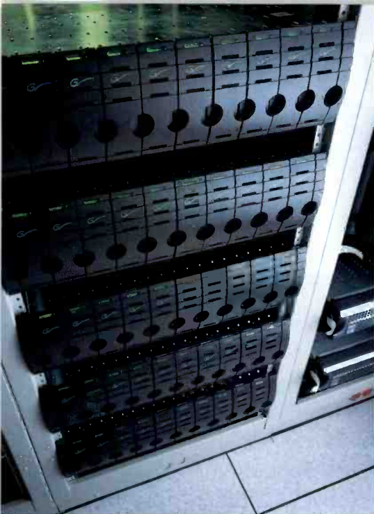
The Thomson Grass Valley media platform servers feature a Fibre Channel-attached RAID storage system.
