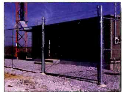
A chain-link fence topped with barbed wire can effectively deter casual would-be intruders. (Photo courtesy of Andrew Corporation.)
