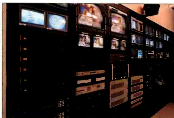
The KAZ-TV master control room features Leitch VR 440 video servers and the Integrator routing system, and Scientific-Atlanta MPEG-2 encoding gear.
