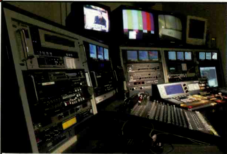
KAZ-TV's production studio in Phoenix consists of an SDI video and stereo analog infrastructure featuring Ross Synergy Series switching. The facility also features Ikegami cameras and Wohler monitoring equipment.
