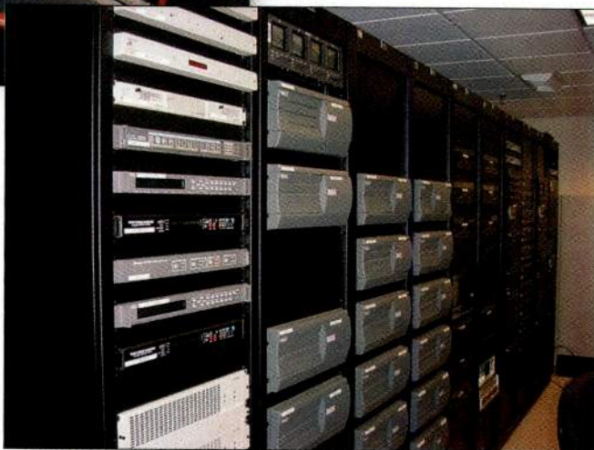
Racks of Pinnacle DekoCast systems, installed in the new Starz Encore operations center, are used to automate interstitials, bug insertion and other on-screen branding.
