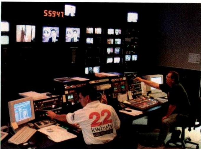
The Thomson Grass Valley M-2100 master control switcher, installed at KVEA-TV in Los Angeles, offers multi-channel operation, extensive keying flexibility, separate and embedded internal digital-audio processing, and a wide range of software-enabled options.
