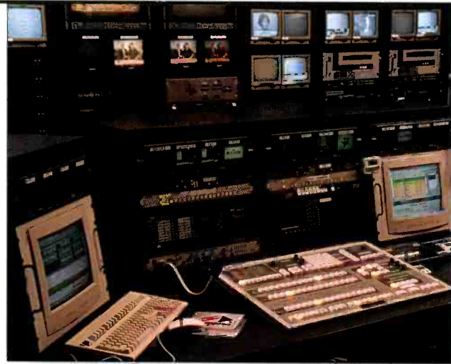
The Leitch Opus and Sundance automation are the key ingredients of the master control console for KAZ-TV in Prescott, AZ. This control room utilizes an embedded SDI infrastructure.
