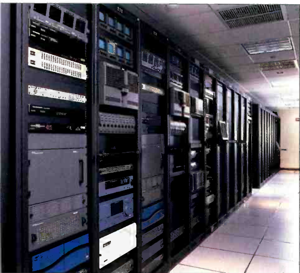
The machine room shown above contains the core infrastructure for Court TV's network operations center, including a Thomson Grass Valley Trinitix 256x256 SDI router, a Sun Microsystems V880 running AVALON, an LSI Logic spinning disk cache, and Motorola's DigiCipher II transmission platform.
