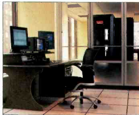
Metadata is attached and media is encoded into a digital format at encoding stations in the facility. The encoded media is then pushed to the archive using AVALONidm software.
