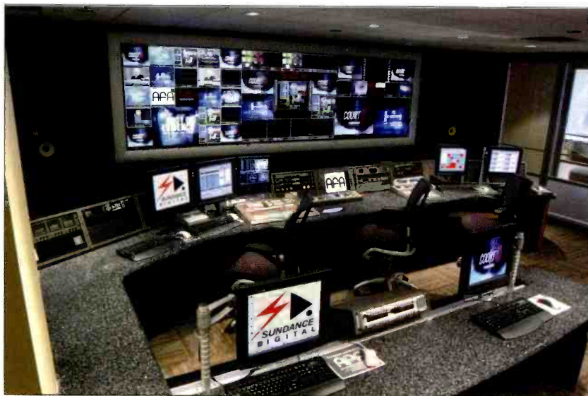
Court TV recently went live from its new digital master control facility in Manhattan, NY, with a fully redundant two-channel Sundance Digital FastBreak automation solution. The system drives three Profile XP video servers: two PVS 1026s for play to air, and one PVS 1044 for ingesting the content. Photo courtesy Court TV. Photo by Andy Washnik.
