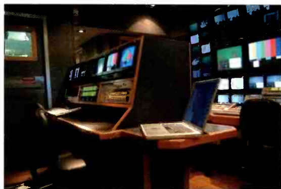
Router control in the production room is handled from a Sony laptop computer on a pullout drawer. The truck's complement is all Sony equipment, eliminating the need for special translation boxes to convert Sony protocol for use with other systems.
