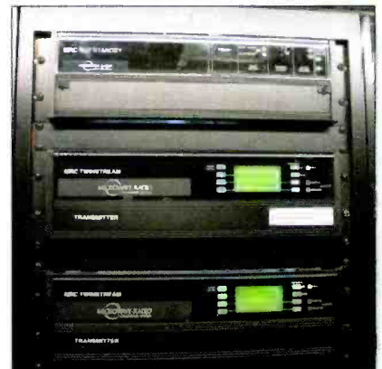
WTVP/WTVP-DT Peoria, IL uses a combined STL system for the NTSC and DTV signals. The hot standby system employs two MRC Twinstream radios. Photo courtesy D.L. Markley & Associates.
