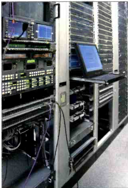
The Grass Valley Encore facility control system from Thomson features tight integration with automation and UM systems.
