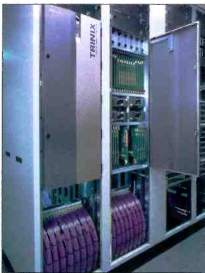
A Thomson Grass Valley Trinix digital routing switcher lets ESPN frame-accurately switch a large number of crosspoints simultaneously.
