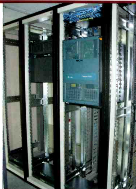
The Catalyst 4500 and 6500 switches provide high-speed Ethernet connectivity for Mediaset's production facilities and individual employees within each site.
