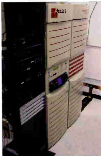
WPSX-DT's 1kW booster in Altoona, PA, is part of the world's first Distributed Transmission (DTx) network.
