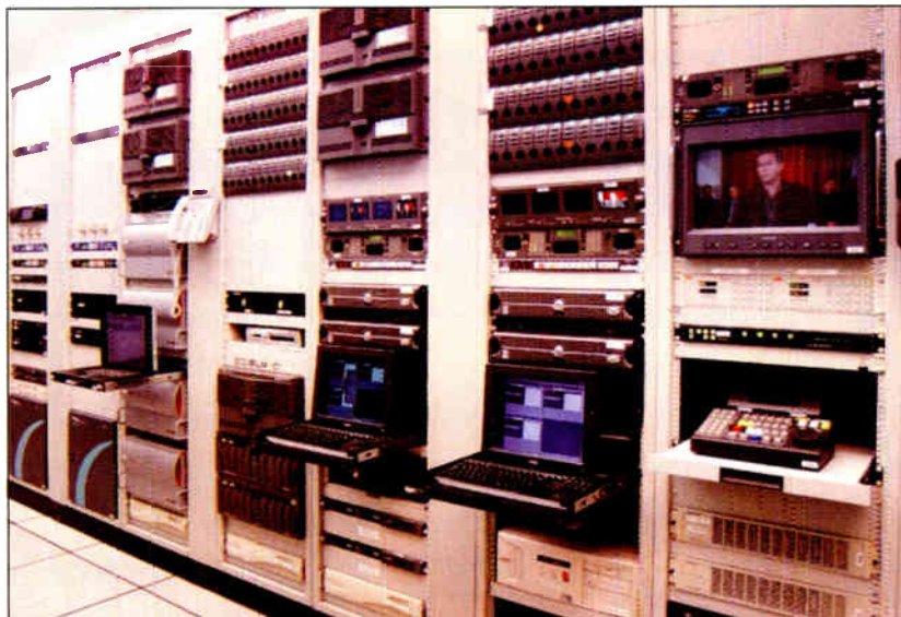
Multiple Grass Valley Open SAN systems from Thomson, consisting of two Profile servers each, hold about four days' worth of content each for four HBO on-air channels. Each movie file is encoded as an MPEG-2 file and stored on hot-swappable Ciprico 146GB drive arrays.
