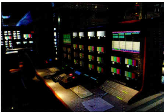
This customized tape production bench has a monitor wall that includes flat-screen and tube monitors but is still only 11in deep.
