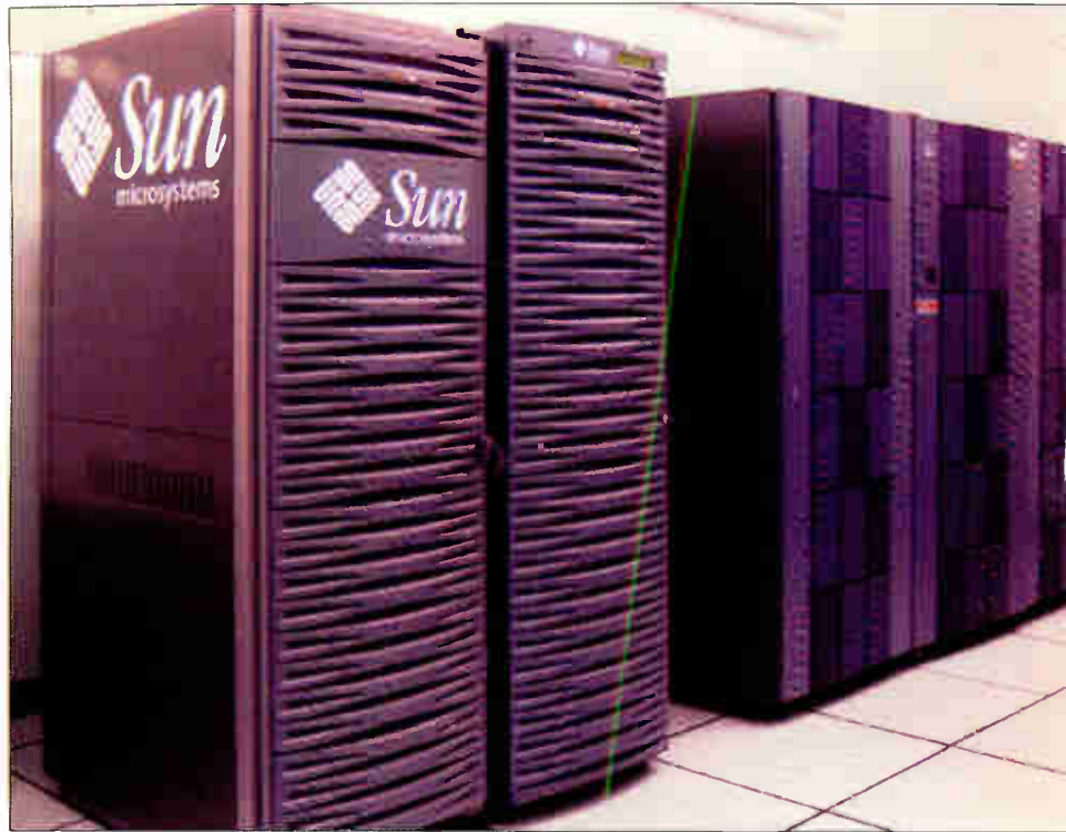
Two Sun Microsystems 6800 series mid-level servers, located on separate floors for redundancy, provide offline storage for approximately one year's worth of content. Content moves between storage arrays at 350MB/s.
