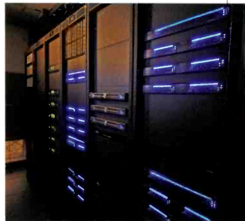
Equipment racks at WCPO-TV house the Omneon Spectrum media server system.
