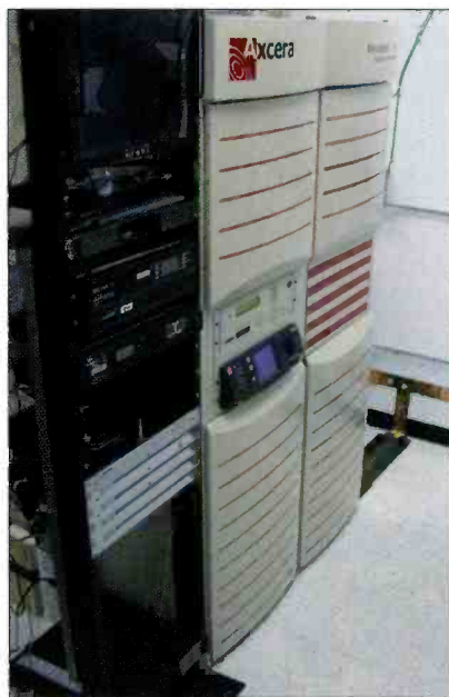
WPSX-DT's 1kW booster in Altoona, PA, is part of the world's first Distributed Transmission (DTx) network.
