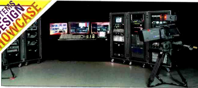
Getting all the equipment mounted into five short racks required careful planning. The equipment above includes a Snell & Wilcox Kahuna 3 ME switcher, Grass Valley Worldcam and Concerto multiformat router and Evertz signal conversion frames.
