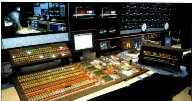
ESPN created resilient, physically dispersed HD-SDI and AES paths to support its HD-originated programming.
