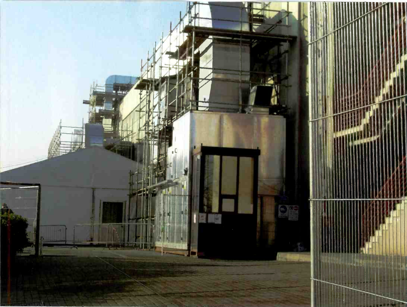
These HVAC systems are installed next to the temporary broadcast facilities at the 2006 Winter Olympics in Torino, Italy.
