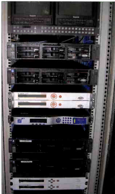
Encoding equipment relies on Thales technology.
