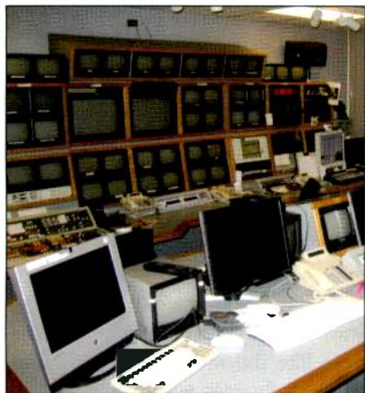
The old Control A was on-air for at least nine hours a day for the last 13 years.
