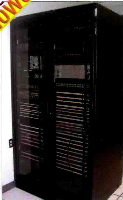
The Pittsburgh control center can even monitor tower lights throughout the entire system.
