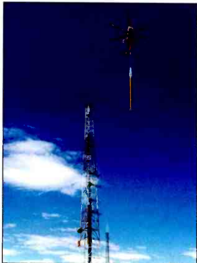
Tower companies should provide a certificate of insurance for liability coverage. Photos courtesy Dielectric.
