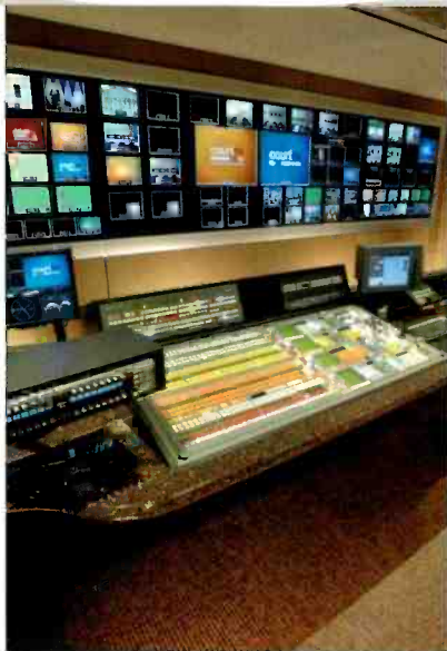
An Evertz remote control panel for monitor reconfiguration sits at the executive producer's position in the middle of the control room.
