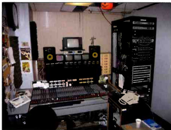
In Court TV's old audio control room, staff members used a Wheatstone SP6.
