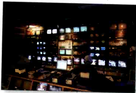
Multiple Leitch X75 multiple-path converter/synchronizers provide the frame-rate conversion for 20 countries.
