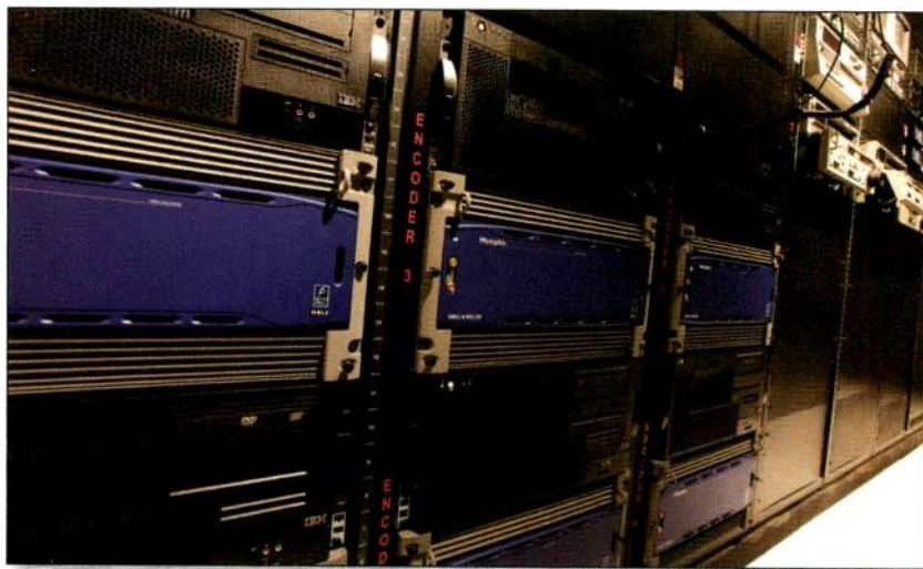
Snell & Wilcox ingest decoders capture high-resolution compressed digital video of NBA games, which are recorded directly into the StorageTek data tape library in real time.
