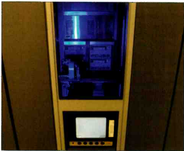
HP StorageWorks tape libraries are used to power Atlas, AMG's digital asset management solution.
