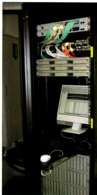
A workstation dedicated to SAN administration makes troubleshooting easier.
