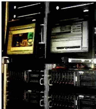
The Discovery Channel uses a 32-channel system for monitoring and logging, with eight Observers (which are located at the bottom of the rack) and one WEB/SQL server (not shown). Photo courtesy of Discovery Channel.
