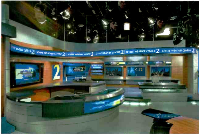
Channel 2, WSB-TV-DT, Atlanta's first DTV facility, transitioned to HD on Sept. 27, 2006. The BDI-designed HD studio played a prominent role in the launch.
