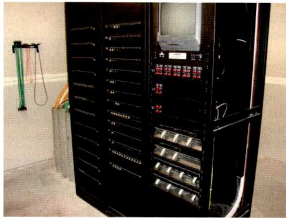
Michigan State University's broadcast control room uses Gepco's coax, triax and audio cables to ensure that broadcasters do not miss a minute of the action on the field.
